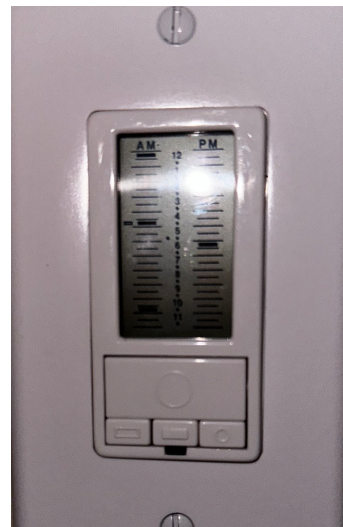
1. automatic fan control; in coat closet.
